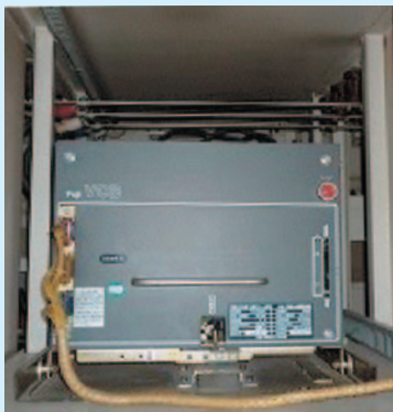
Existing VCB manufactured in 1982
