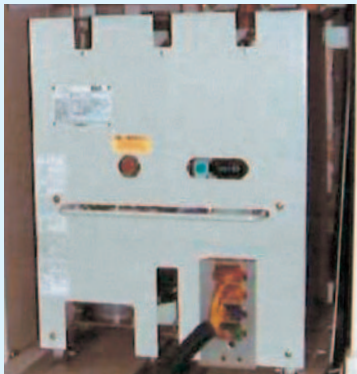
Existing VCB manufactured in 1982
