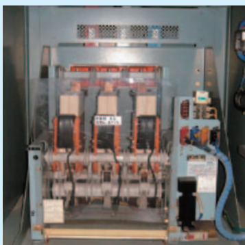
Existing HC23 air magnetic contactor
